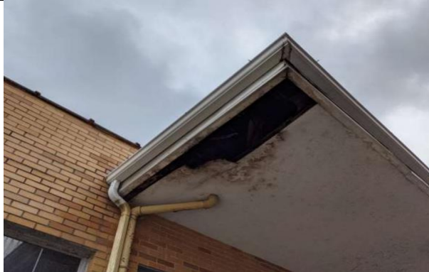
Greyhound Bus Depot, south canopy roof soffit showing deterioration.
