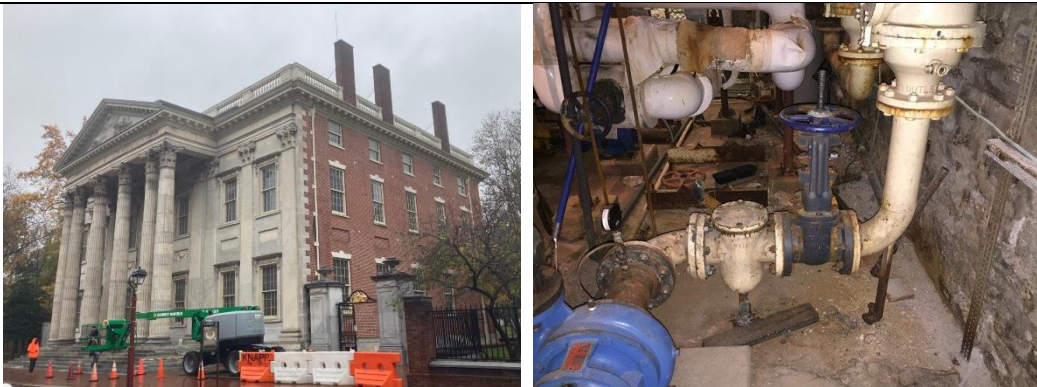
Left: Street view of First Bank of the United States. Right: Outdated and failed building systems decaying in place.
