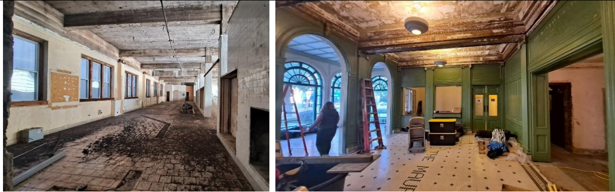
Left: Advanced deterioration in the Libbey Bathhouse. Right: Deterioration in the Maurice Bathhouse lobby.
