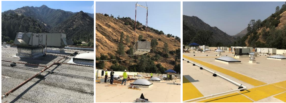
Projects like this one at Yosemite National Park, to rehabilitate the roof and replace HVAC units at the El Portal Maintenance Complex are funded through the Repair and Rehabilitation program. The Maintenance Complex functions as the core administrative site for the park, and houses the facilities management, safety, volunteer, engineering, visitor protection, resources management, and park dispatch offices.
