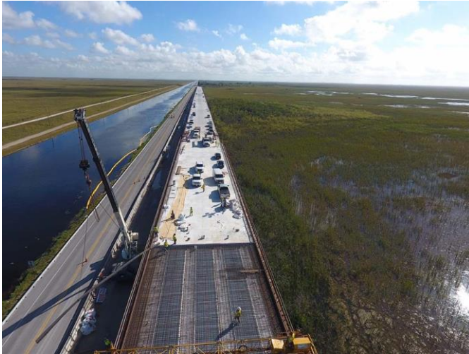
The Tamiami Trail Next Steps Project is enhancing the connectivity and water flow between the marshes north and south of the Tamiami Trail while maintaining the vital transportation link between southwest Florida and Miami.
