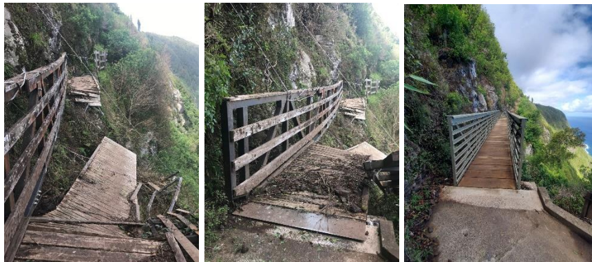
Projects like this one at Kalaupapa National Historical Park, to repair and rehabilitate a flood damaged bridge on the Upper Pali Trail are funded through the Repair and Rehabilitation program. The Pali Trail is the only overland access into the Kalaupapa settlement, and it is used by NPS and State staff that hike to work, by visitors to access the settlement, and by the mule tour operators.
