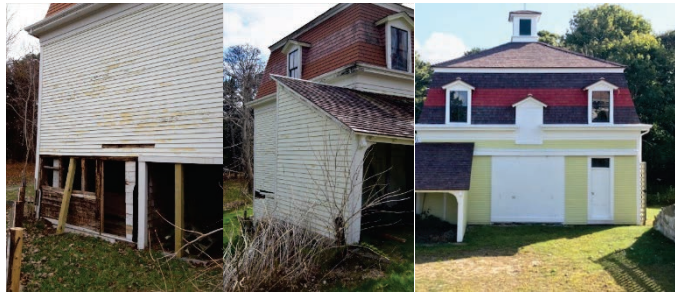
Projects like this one at Cape Cod National Seashore, to repair and rehabilitate the deteriorated Captain Penniman House Barn are funded through the Repair and Rehabilitation program. Constructed in 1868, the facility is a National Register property and is a centerpiece of the Fort Hill Rural Historic District.
