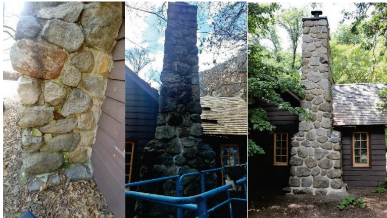
Projects like this one at Yosemite National Park, to preserve external stone chimneys on Valley Residences, are funded through the Cyclic Maintenance program. Built in the 1920s and 1930s, the historic residences are contributing features of the Yosemite Valley Historic District and are listed on the National Register of Historic Places.
