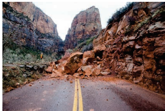
One of several major rockfalls affecting Zion National Park's road and trail system. (NPS Photo)
