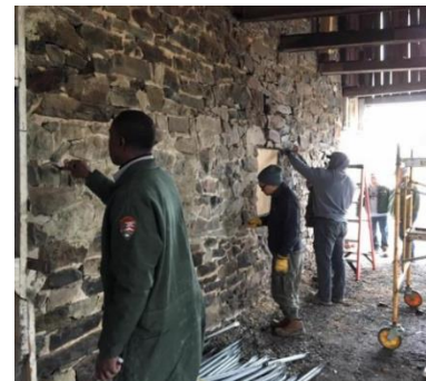
NPS employees providing training in the maintenance and restoration of historic masonry. Students included a veteran cohort of the Traditional Trades Apprenticeship Program at Gettysburg NMP.
