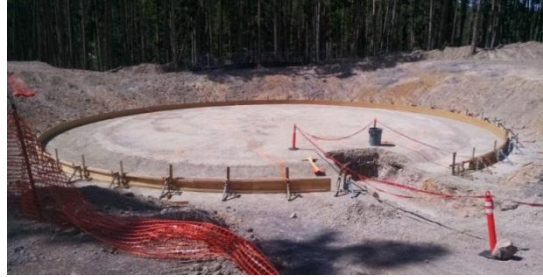
Foundation for a required storage tank associated with the Fishing Bridge waterline
