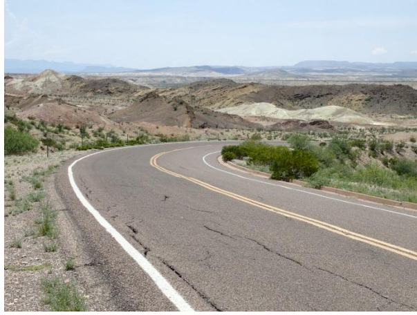
A curve in the road at Big Bend NP shows cracking.
