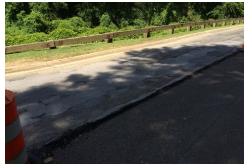
Road condition on the George Washington Memorial Parkway
