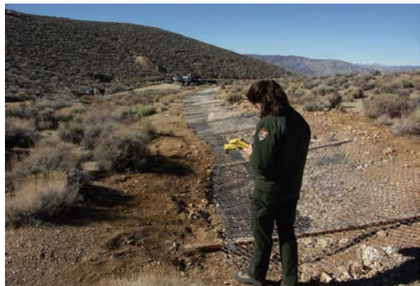
An open slope was closed with cable nets and wire mesh at Skidoo Gold Mine. Death Valley NP. California.
