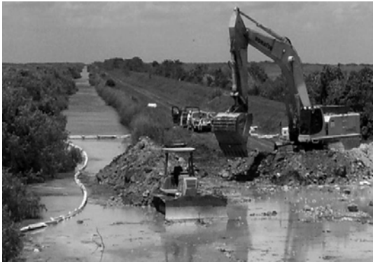
Degradation of the L-67 extension canal and levee to improve hydrologic conditions of Shark Slough
