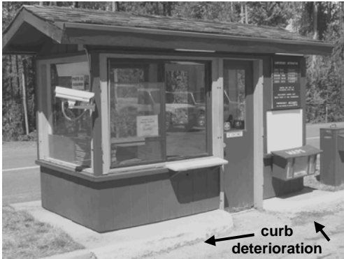
General deterioration of the entrance station building; entrance building condition lacks protection from vehicles.
