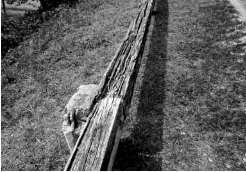
Rotting timber guardrails cannot withstand vehicle impact and provide a false sense of security.
