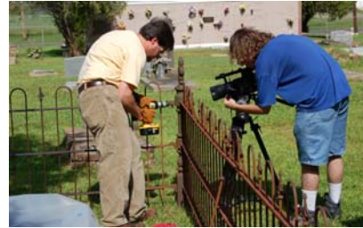
Jason Church, NCPTT materials conservator, demonstrates the proper method to remove a broken bolt during filming of the Basics for Iron Fence Care video. (Stace Miller)
