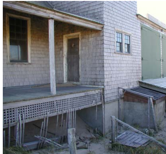
Deteriorated condition of Old Harbor Life-Saving Station (exterior) at Cape Cod NS.
