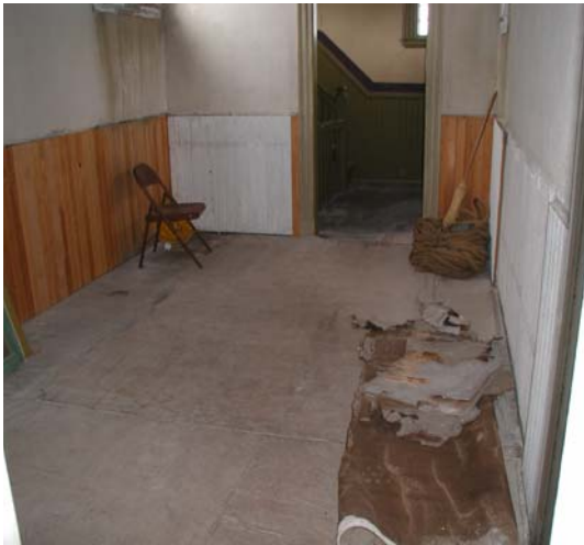
Deteriorated condition of Old Harbor Life-Saving Station (interior) at Cape Cod NS.
