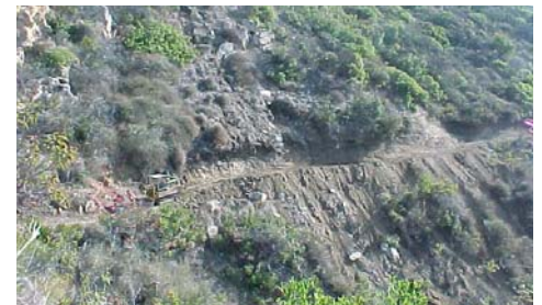
After: Repairs were completed and the asset is now maintained in "good" condition.
