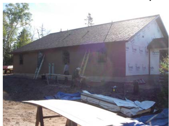
Construction of one of the new units that will replace the houseboat and a trailer unit at Isle Royale NP.
