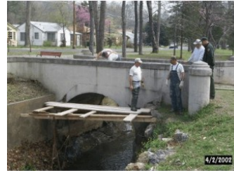
Rehabilitation of unsafe foot bridges within Whittington Park at Hot Springs NP
